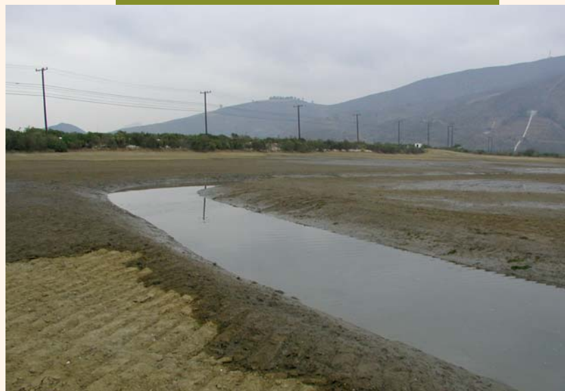
The beginning of construction that incorporates sewage sludge into the restoration of Mugu Lagoon in Ventura County, Calif., and the restored wetland at the beginning of its “life.”
